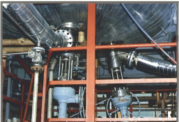
TITANIUM TANK BOTTOM ANGLE VALVES OPERATING ON HIGH TEMPERATURE PTA REACTOR.
